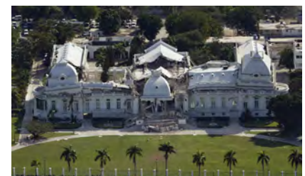
Figure 1: The damaged National Palace is an iconic image associated with the earthquake.
