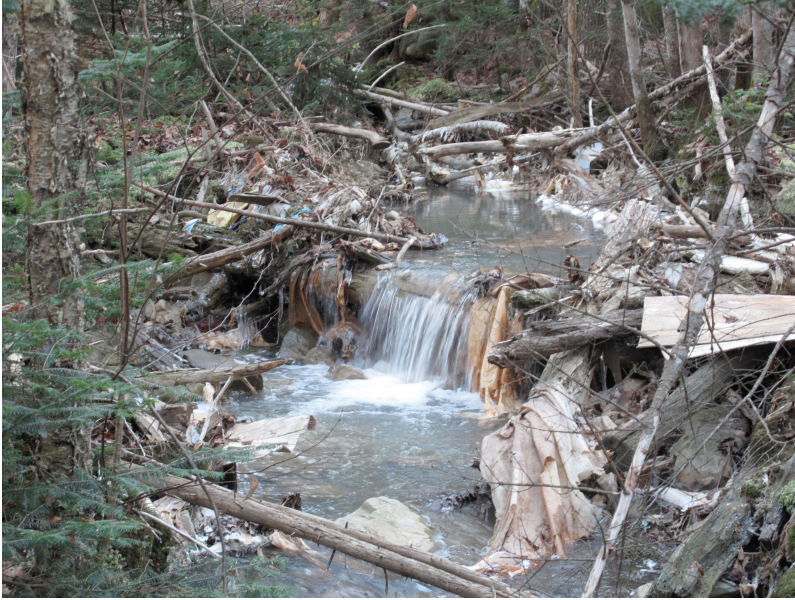
Figure 4.12: N 44° 39.589 W 063° 40.613. Plastic garbage and cloudy water in the stream flowing from the culvert under the corner of Lacewood Drive and Highway 102. Jennifer MacLatchy, 2013.
